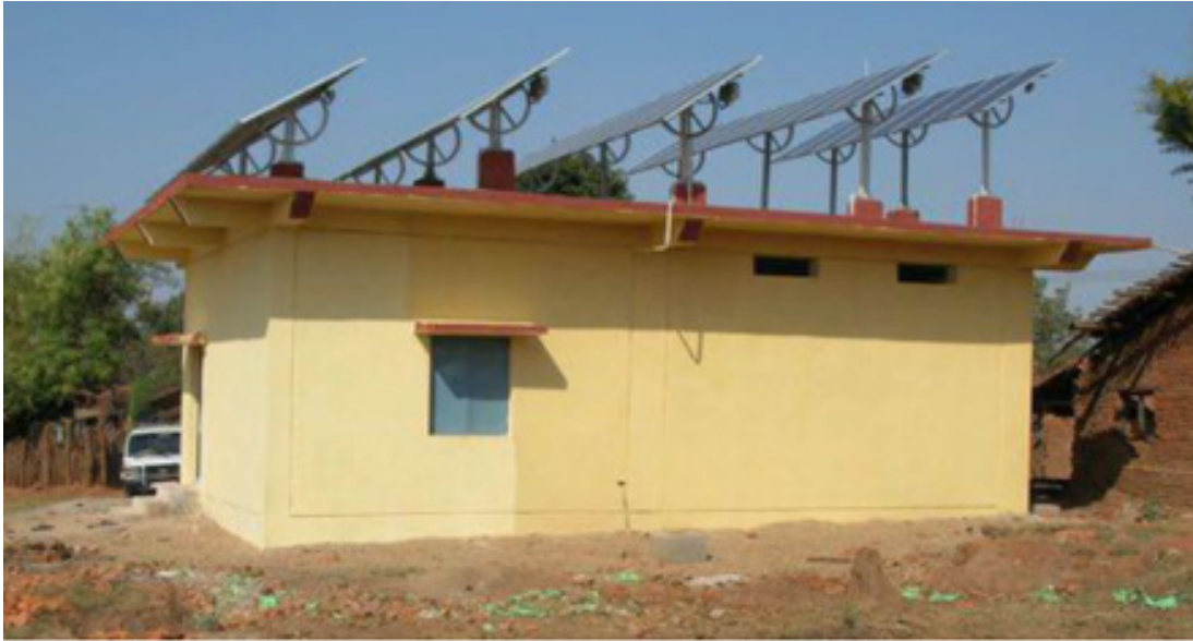
array installed on a roof of the control room
